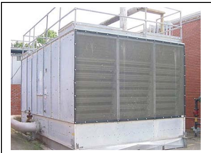
Cooling Tower Filters
