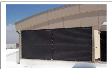
Louver Intake Filters
