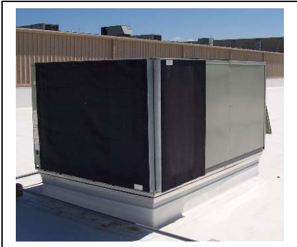
RTU Filters & Hail Guards
