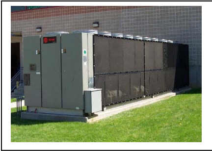
Chiller Coil Filters
